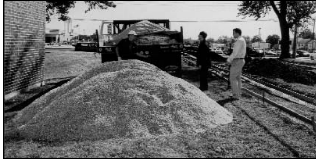
Howard Worcester, recycling coordinator, delivers recycled glass from the Truman Recycling Center for the sand base of a four-foot wide concrete sidewalk, one part of an energy trail connecting the Senior Wellness and Community Center to A.T. Still University's Thompson Campus Center. Aesthetically, the trail will appear as a concrete sidewalk, but beneath the surface the glass base will provide a sturdy foundation for walking and enjoying outdoor exercise.
